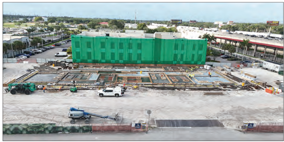
HOLLYWOOD CONSTRUCTION: Aerial views on April 16 provide a glimpse of major construction projects on the Hollywood Reservation. Above, the senior center; middle, Betty Mae Jumper Medical Center expansion; and bottom, the community center, which will be built on the site of the Estates Clubhouse, which was recently demolished.
