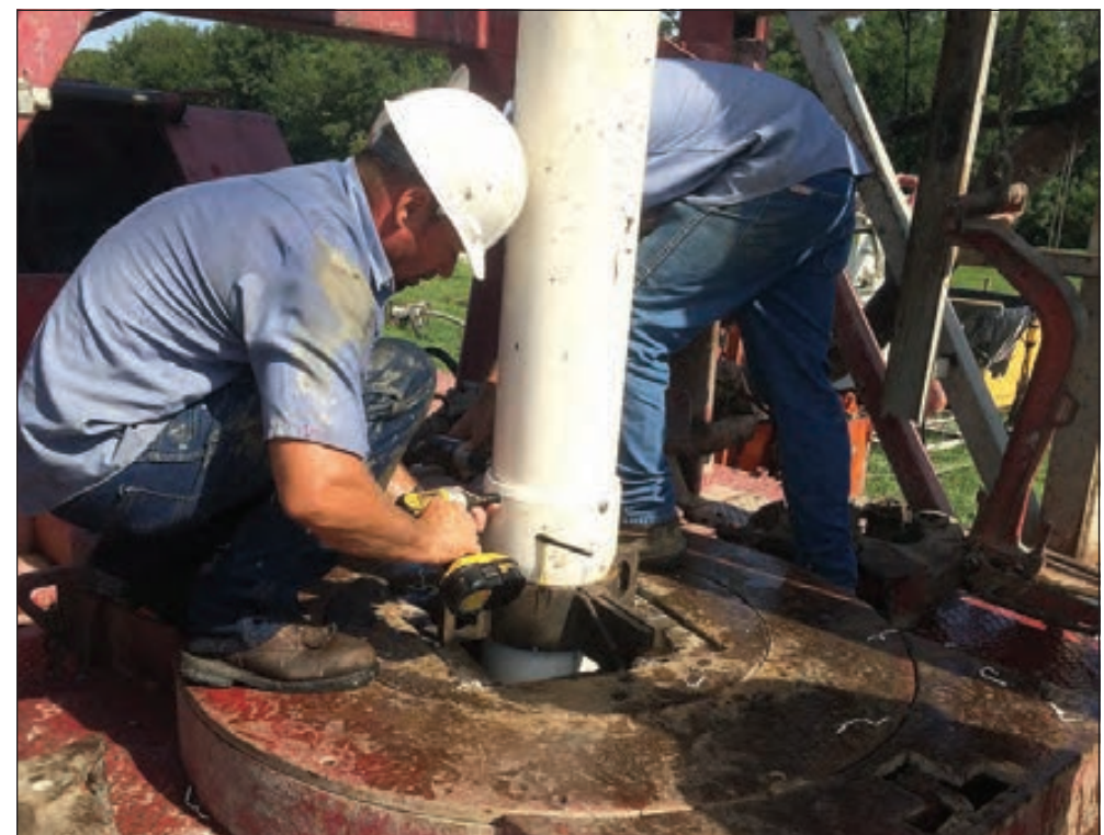
Workers install the production casing on one of the new wells that tap into the Upper Floridan Aquifer in Brighton in April 2015. The well will draw water from about 675 feet below the surface.
