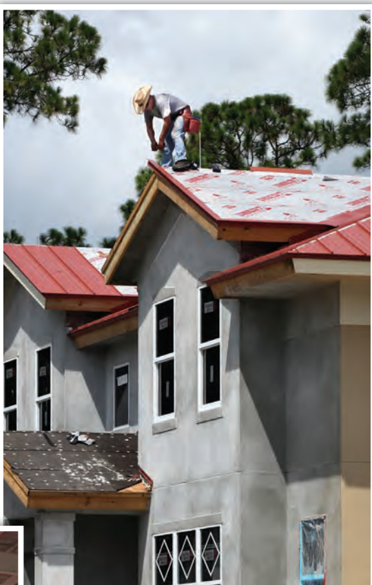
HIGH AND TIGHT: A carpenter works on a roof July 30 at the Big Cypress townhomes construction site on Eloise Osceola Street on the Big Cypress Reservation.
