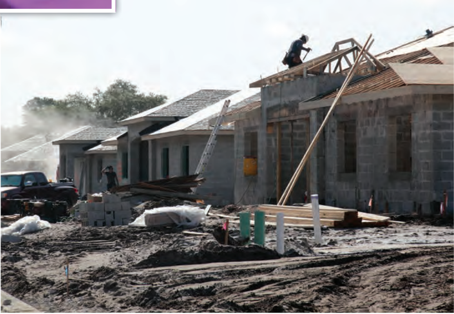
HOME SWEET HOMESITE: The Hollywood Reservation is abuzz with construction activity as eight homes are being built across from the Howard Tiger Recreation Center.
