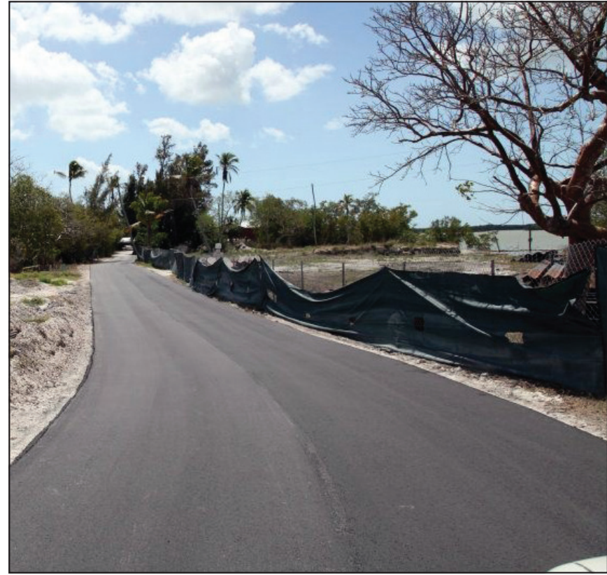
Peter B. Gallagher Florida Georgia Grove began repaving Mamie Street, complying with a September 2011 court order.
